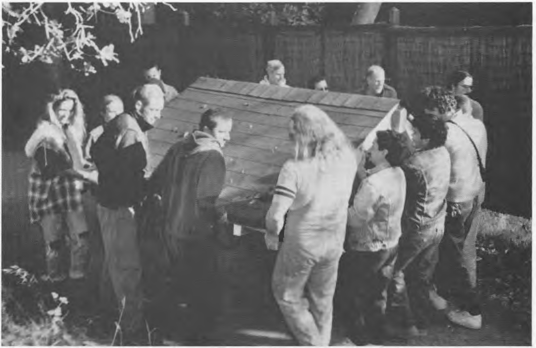
A group of Tassajara residents and members of the deconstruction crew moved the entry roof from the women's side of the baths across the creek in one piece.
